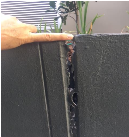
Ground movement, not from construction but from lack of moisture in soil below building.
